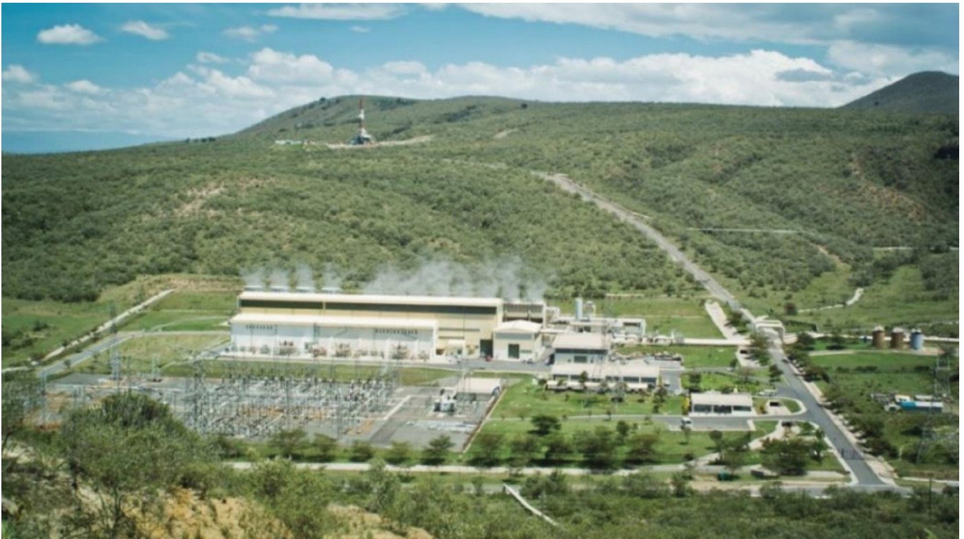
Olkaria Geothermal Plant
