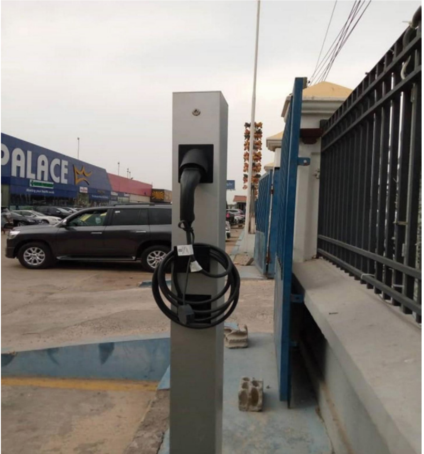
Porsche Charging Station located at Palace Mall, Spintex
